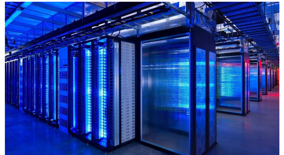
Multi-Node Supercomputer connected over PCI buses
